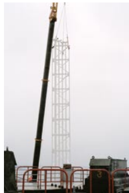
The 80-foot vent mast, which enables venting of gaseous elements, was repaired, painted and returned to its position at starboard side aft on the Launch Platform.
