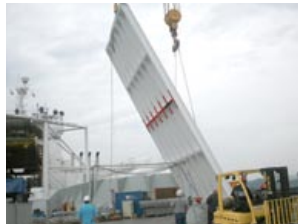
Work on the hangar included repairs to the roof and doors. Here, the aft hangar doors are re-installed on their tracks.
