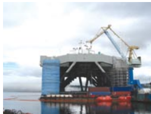
Activities at the shipyard required large cranes, substantial scaffolding and a variety of specialized work crews.
